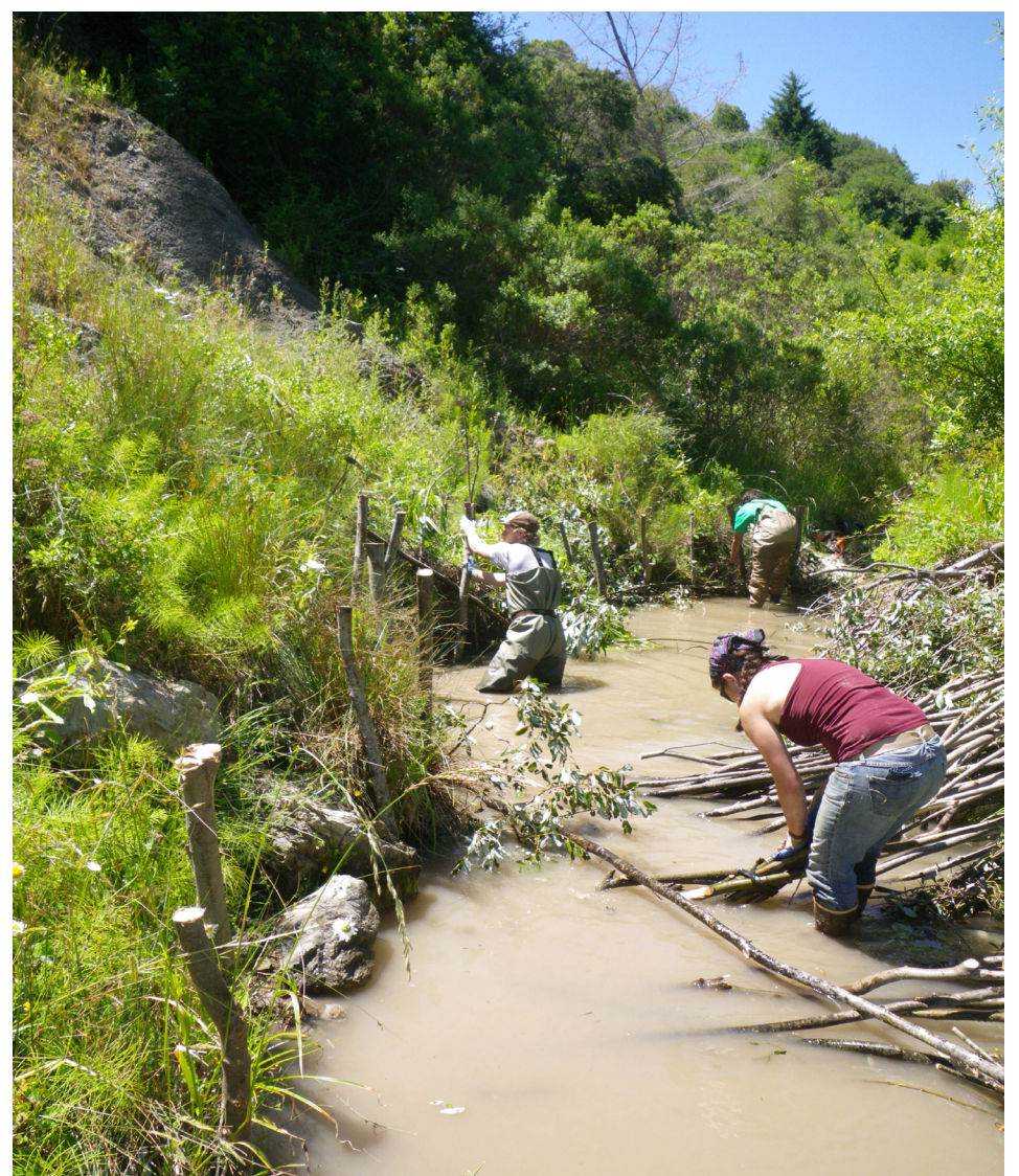
Below: RER crew installing a willow fence on Granny Creek. Photograph by Hugh McGee
