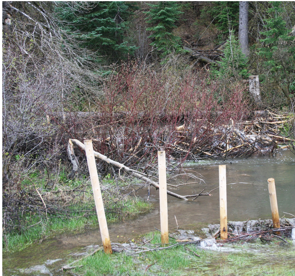
Above: A Beaver Dam Analogue (BDA) consisting of pounded posts interwoven with vegetation and sealed with locally sourced clay. Similar structures will be created in the McKee Creek Watershed. Photograph courtesy of Elijah Portugal, Redwood Community Action Agency.
