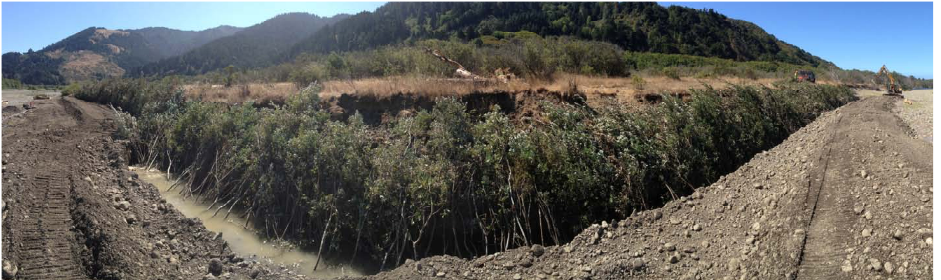
Completed trenched willow baffle site in the Mattole Estuary. Photograph by Hugh McGee
