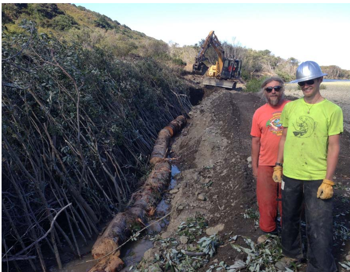
Above: John Summers and Bob Anderson assist with a trenched willow site. Wood is placed in groundwater at the base of the willow cuttings in order to provide dry-season moisture for rooting willows, as well as structure to the trench.
