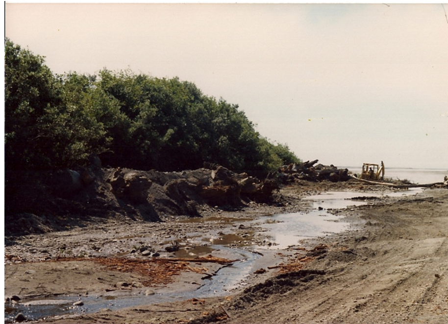
1991: Revetment structures placed along south bank. All photographs courtesy of Michael Evenson unless noted.
